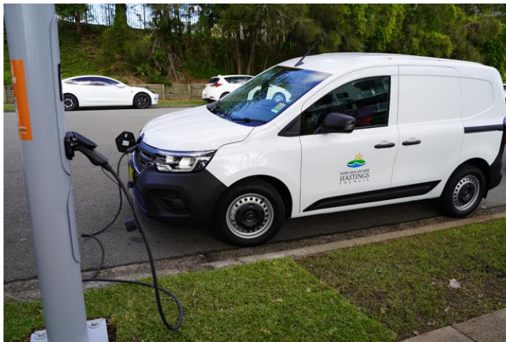
Image 2 - Council EV utilising the Streetlight EV Charger
